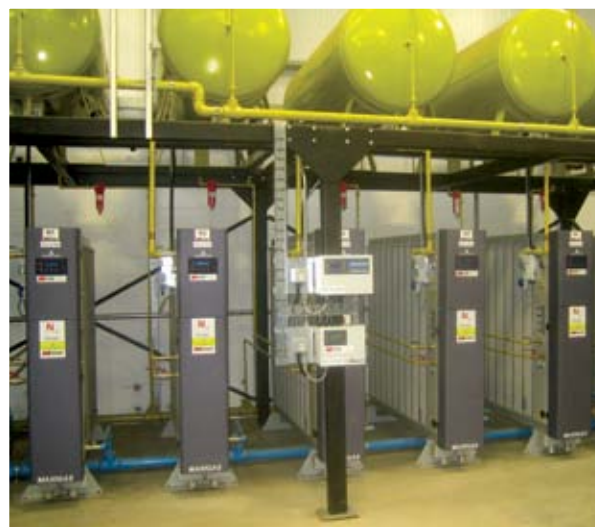
A six bank MAXIGAS installation, (five generators in view) satisfy the peak demand, each capable of supplying 20% of the output. The banks cascade on and off load as the flow varies with factory production requirements. This saves significant energy costs during low flow periods, in the form of lower compressed air demand. The sixth bank provides 100% back-up and allows for 100% up-time during maintenance.
